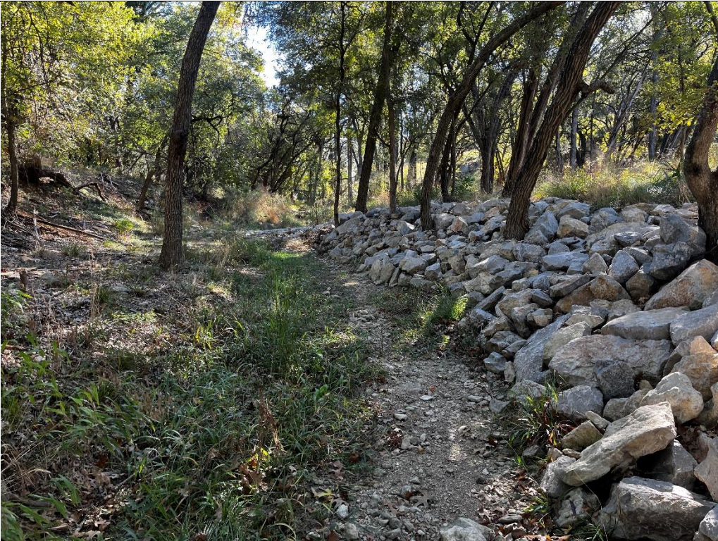
Photo 10. Stabilized infrastructure between grade control structure # 5 and #6, facing downstream. Photo taken on 11/21/2024.
