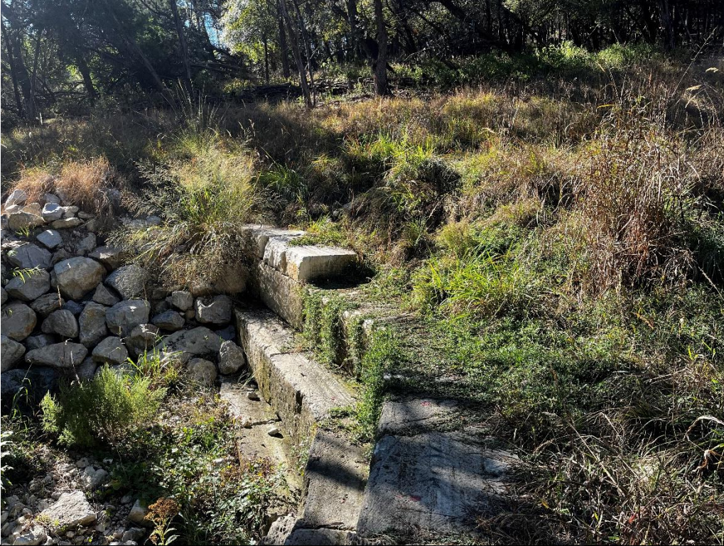
Photo 9. Grade control structure #6, vegetation established in-channel and along banks. Photo taken on 11/21/2024.
