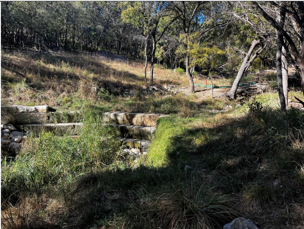
Photo 8. Station 8, between grade control structure #5 and #6, facing upstream towards Sessom Creek and Windmill tributary confluence. Photo taken 11/21/2024.
