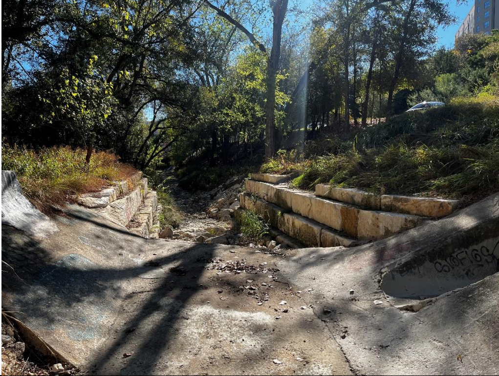
Photo 3. Station 3, directly downstream of gully control #1 and #2, facing downstream. Photo taken 11/21/2024.
