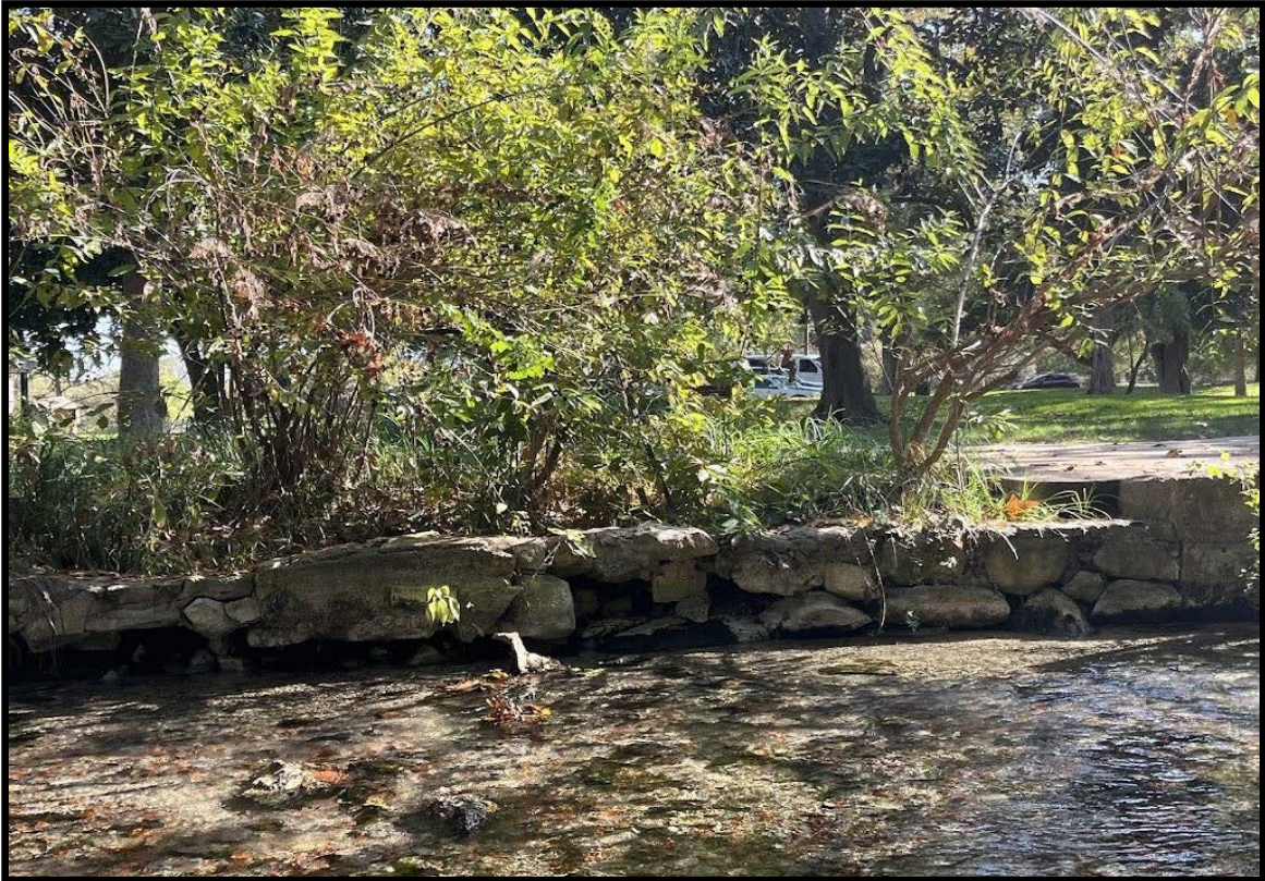
Figure 3. Low water levels have undermined several portions of the rock wall along Spring Run 3. Some areas of the wall have completely caved in undermining vegetation roots. Areas like this are susceptible to collapse and further erosion.
