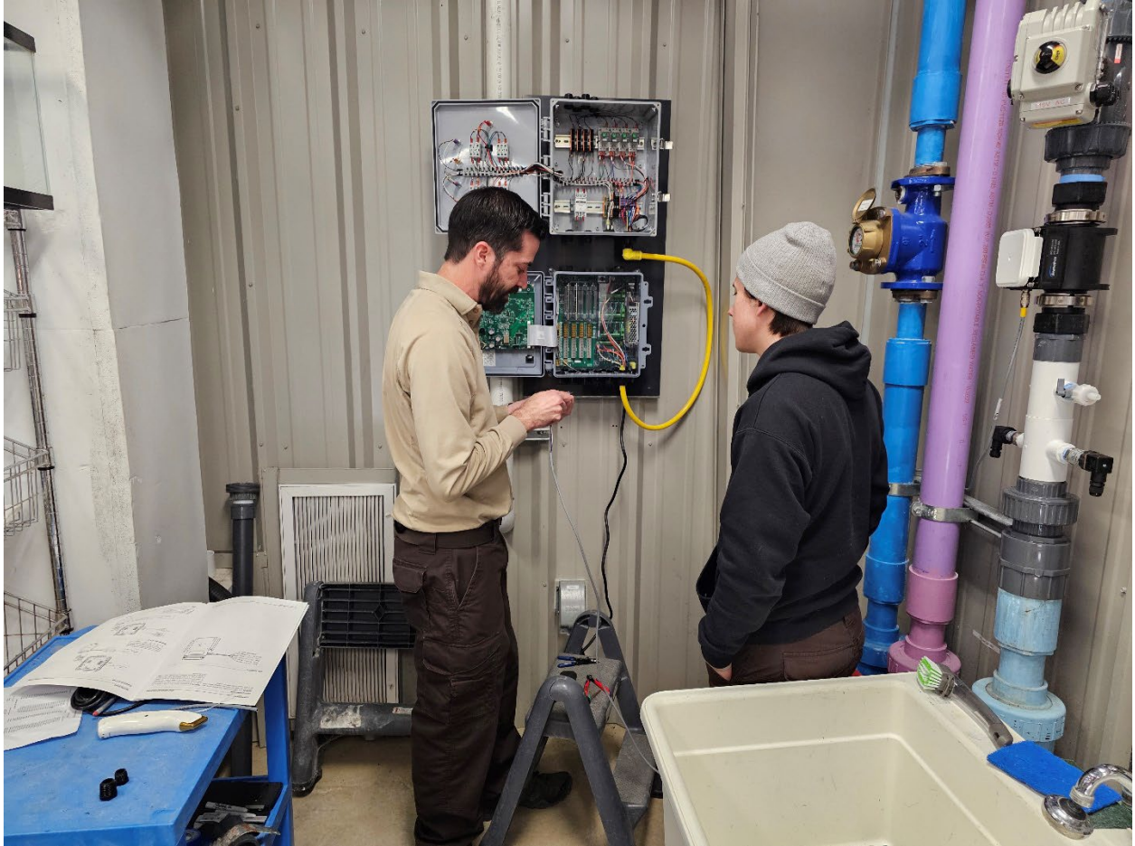
Figure 2. Daw provided demonstrations of sensor wiring to Shawn Moore.
