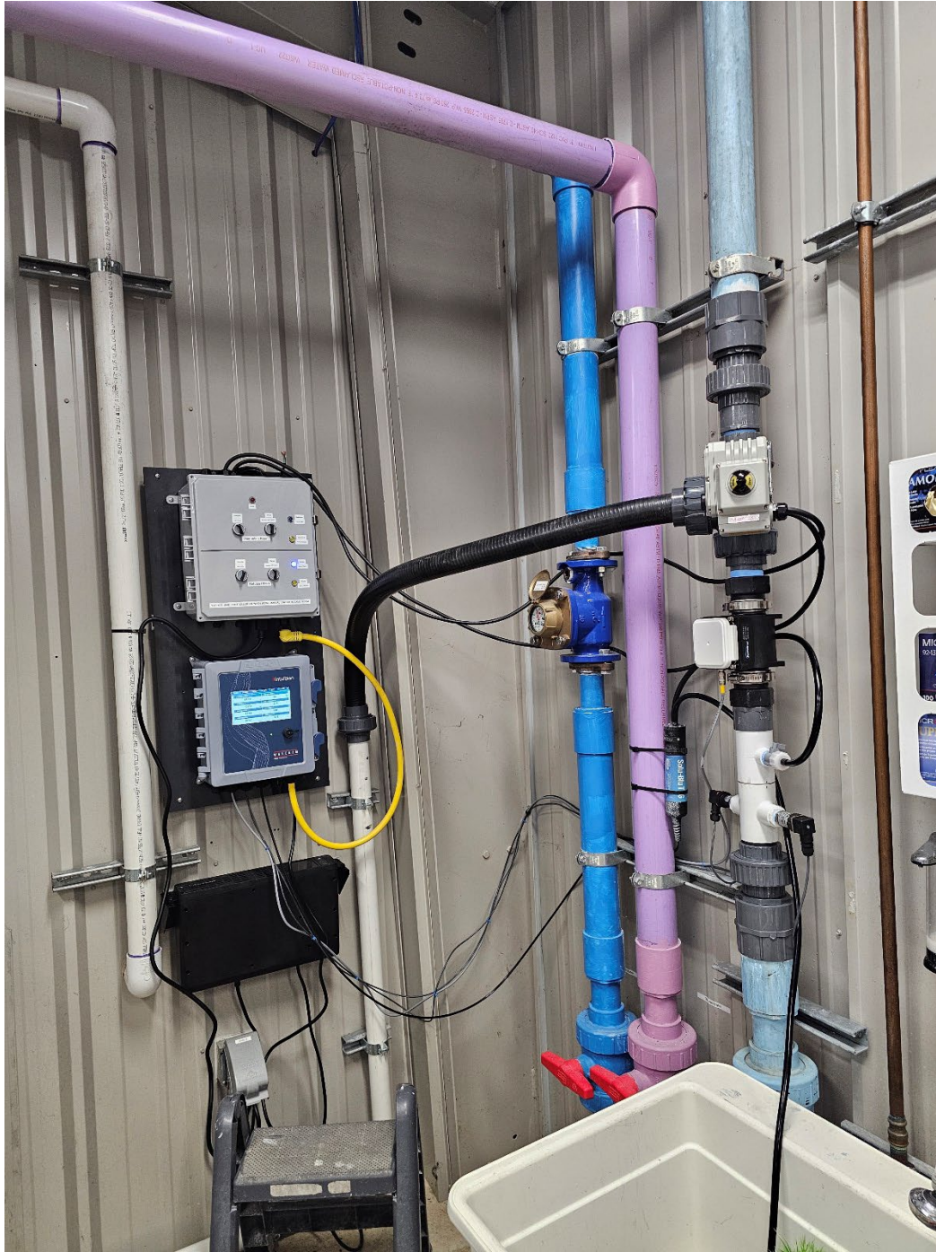
Figure 3. The completed first phase of the supersaturation diversion project in the SMARC refugia. The system affords further security using an uninterruptable power supply (UPS). Supersaturated water is directed into trench drains.
