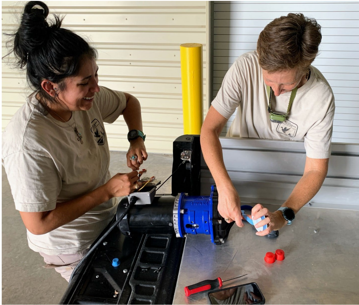
Figure 1. Dominique Alvear (left) and Heidi Meador (right) wiring and preparing a new pump to be replaced on a Refugia tank.
