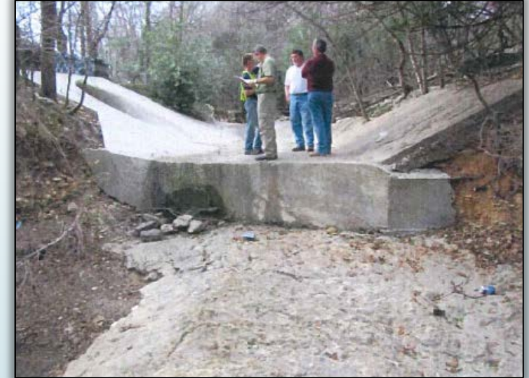
Scour hole below drop structure – Site of RPS project #9 (RPS photo)
