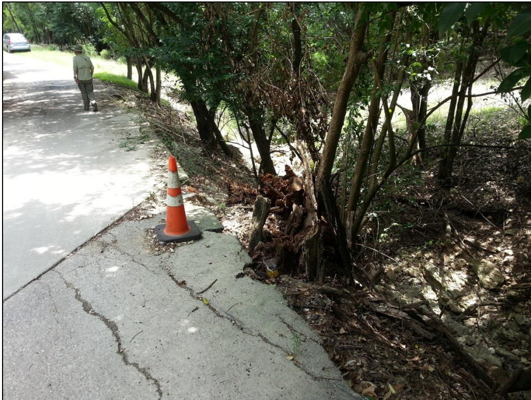
Figure C3. Canyon Road threatened by stream erosion in Reach 2
