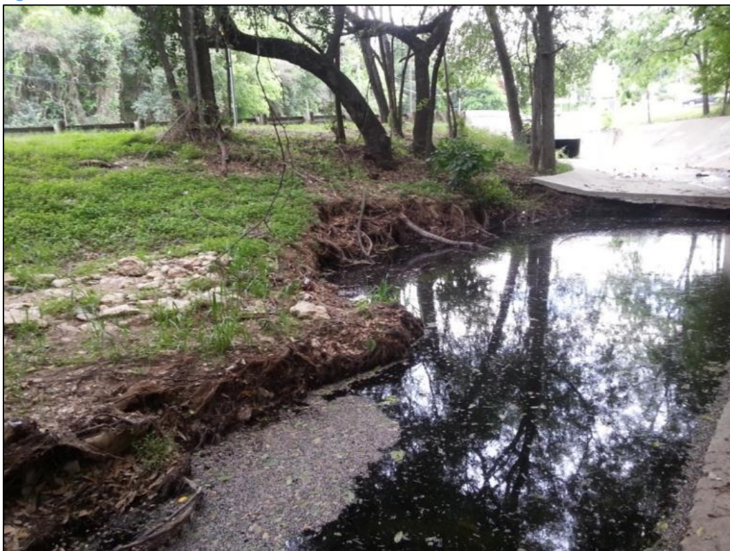
Figure C10. Bank erosion and undermined concrete channel bed in Reach 1
