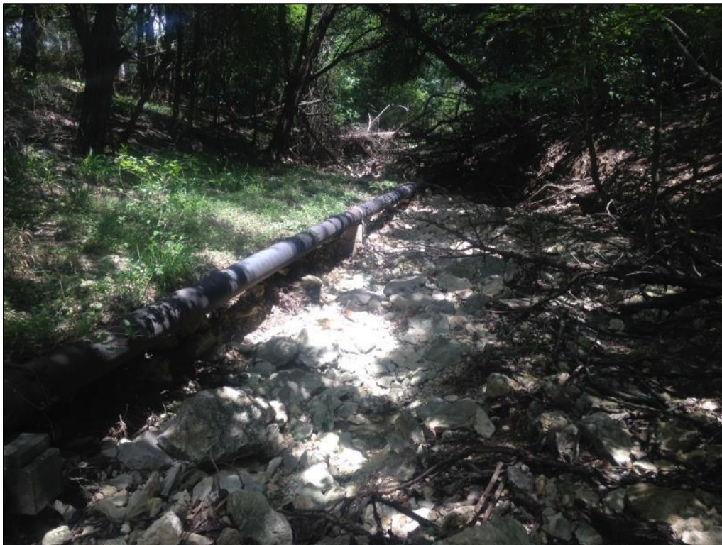
Figure C2. Threatened wastewater line in Reach 2 above the Loquat-Canyon intersection
