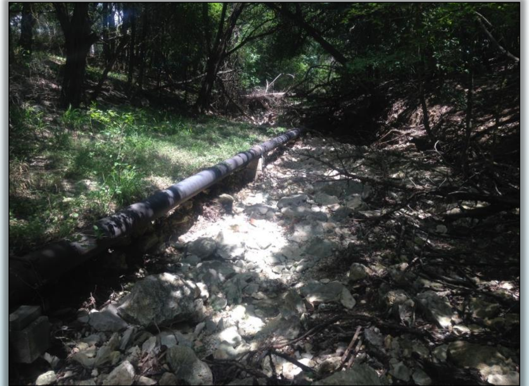
Threatened wastewater line in Reach 2 above the Loquat-Canyon intersection
