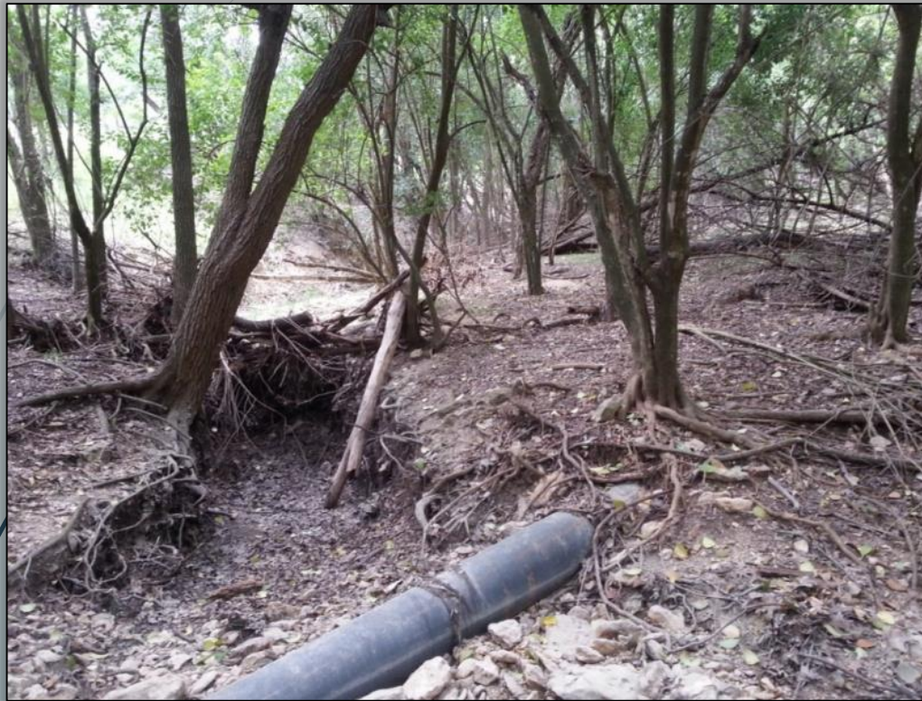
Bed and bank erosion with exposed wastewater line in Reach 2
