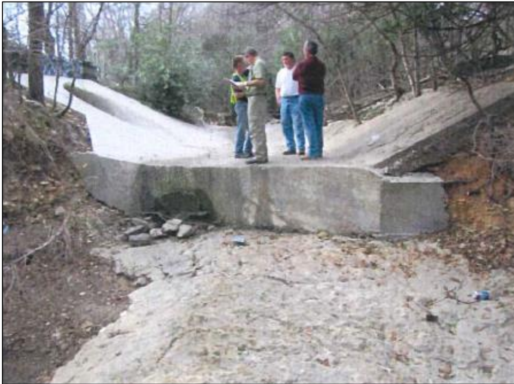
Figure C7. Scour hole below drop structure – Site of RPS project #9 (RPS photo)
