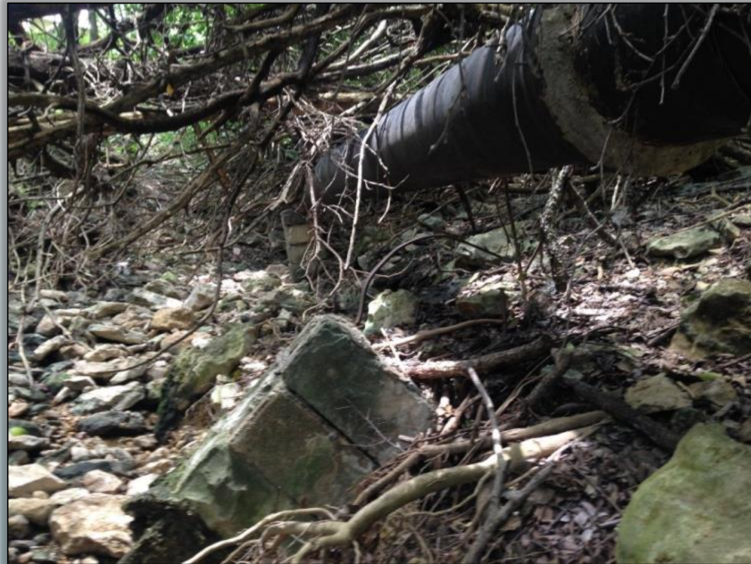
Collapsed wastewater line support in Windmill Tributary
