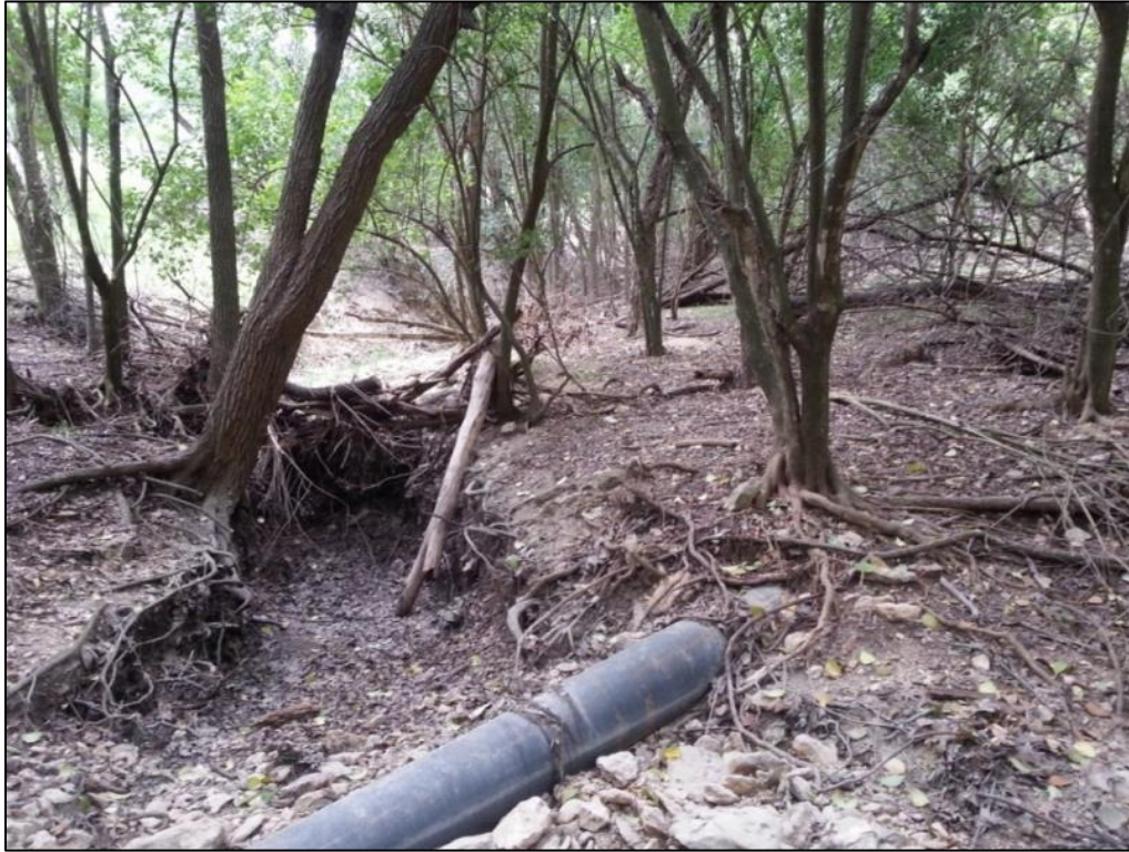
Figure C1. Severe bed and bank erosion with exposed wastewater line in Reach 2
