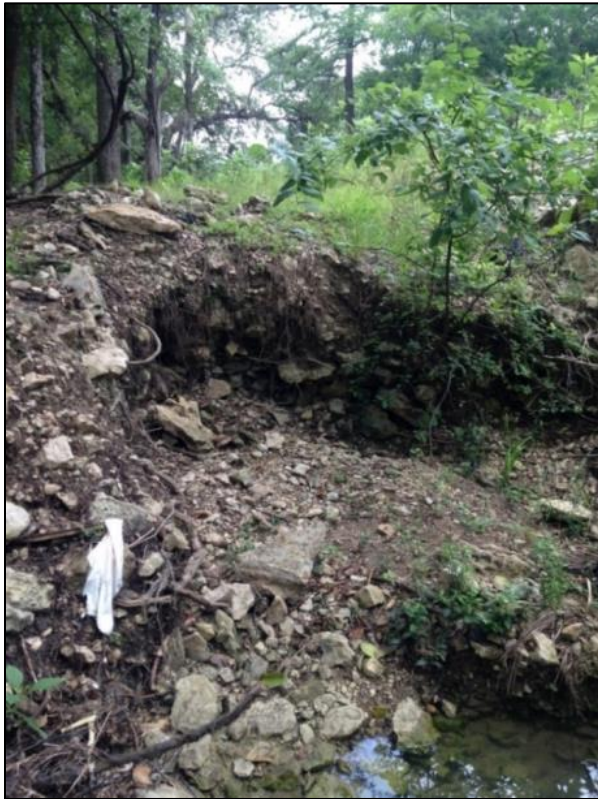
Figure C11. Bank failure in Windmill Tributary
