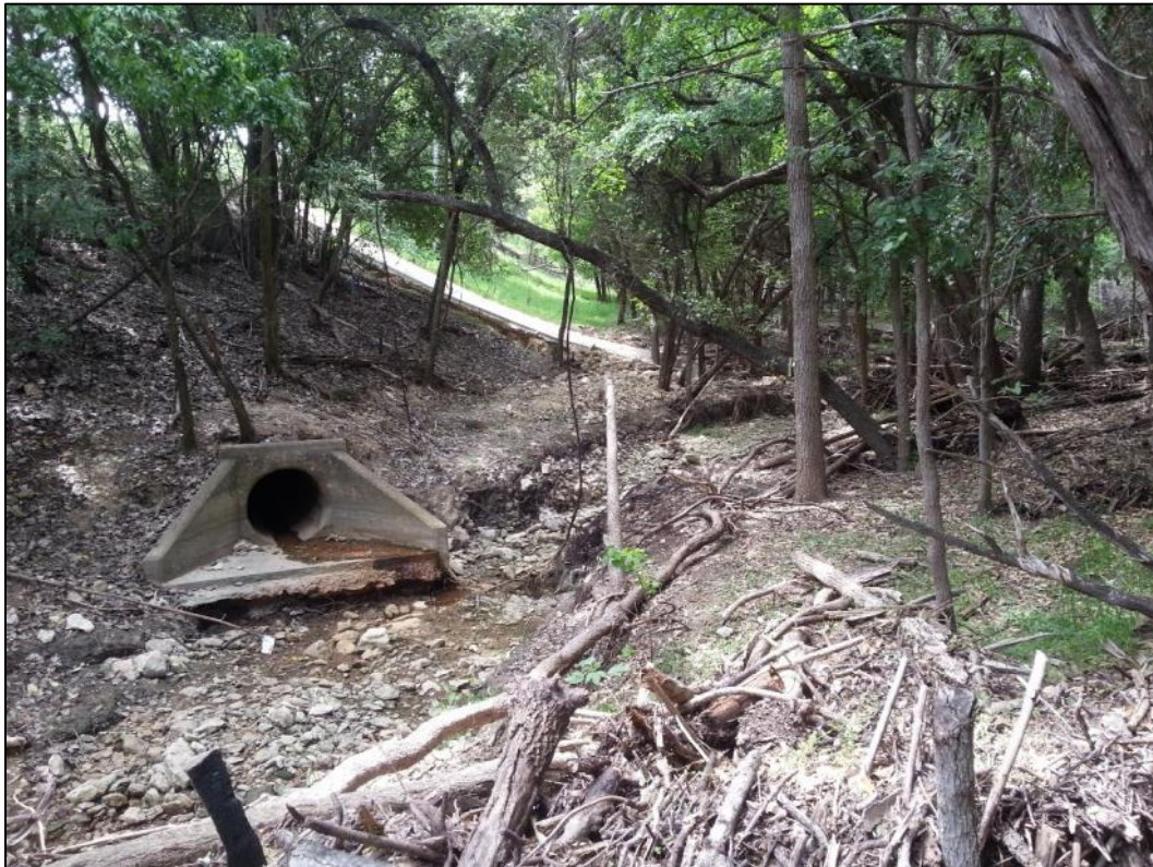
Figure C6. Eroding and erosive outfall from “The Gulch” tributary near RPS project #10 site
