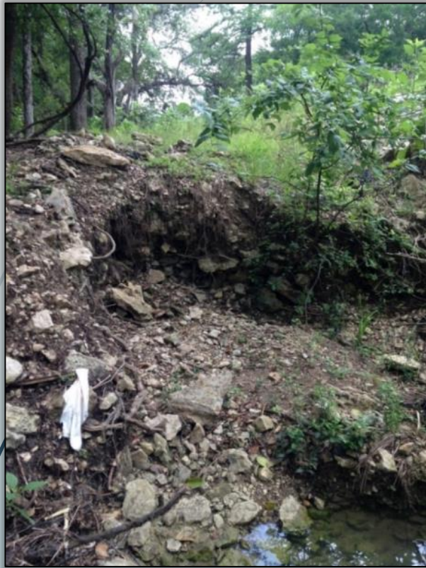
Bank failure in Windmill Tributary
