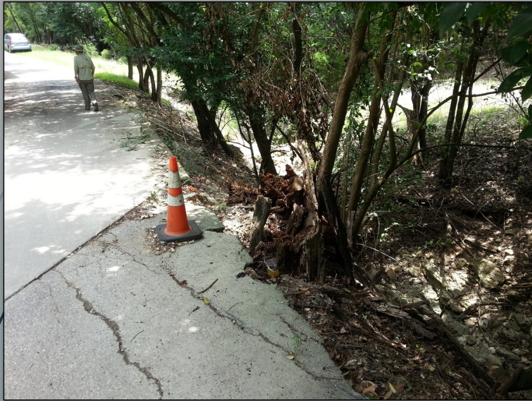
Canyon Road threatened by stream erosion in Reach 2
