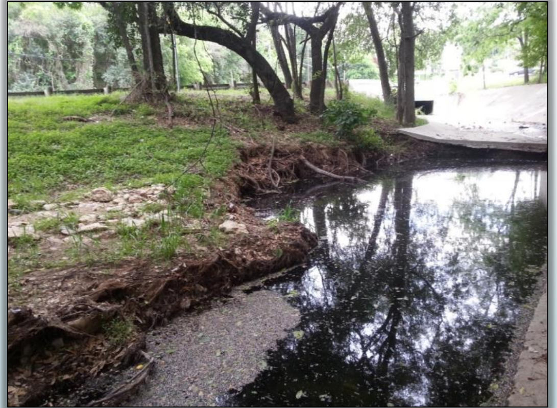
Bank erosion and undermined concrete channel bed in Reach 1
