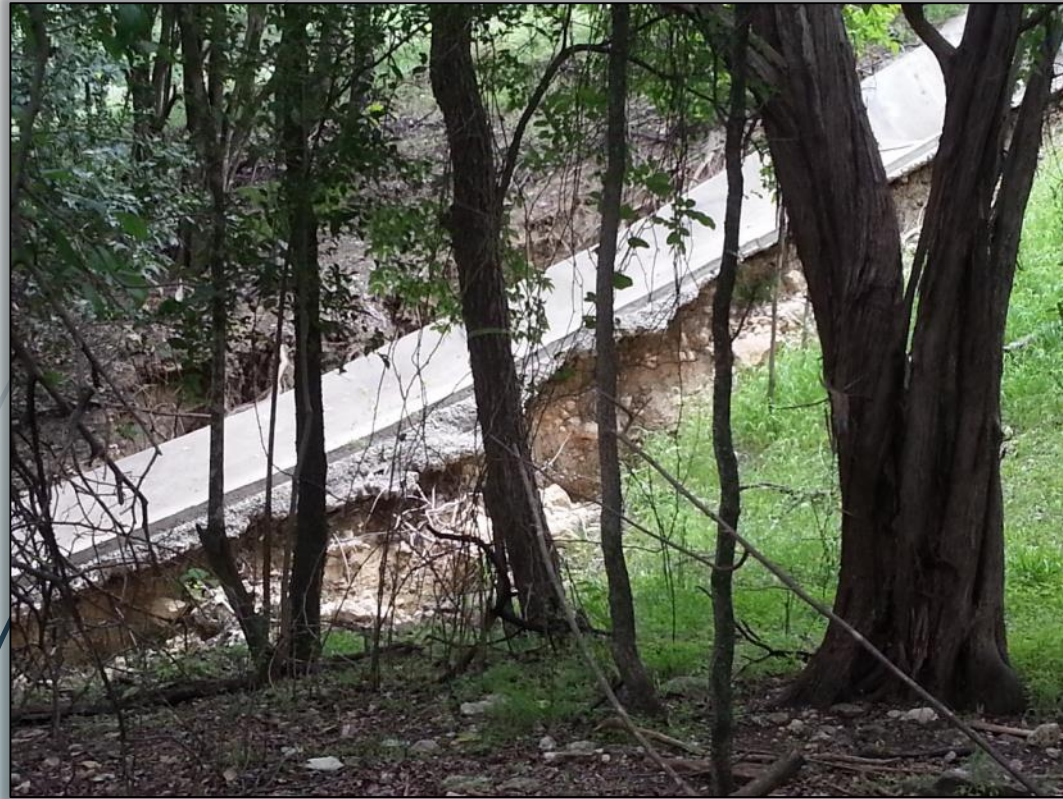
Severely eroded flume at TX ST outfall – Site of RPS Project #10
