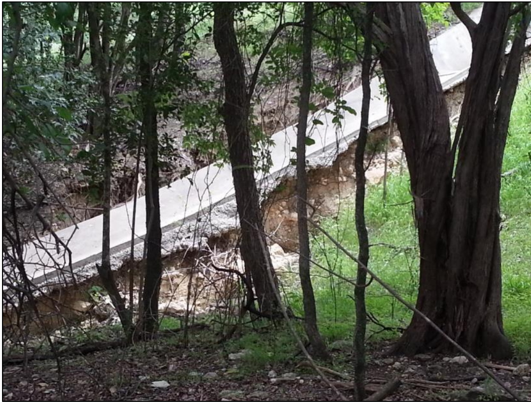
Figure C5. Severely eroded flume at TX ST outfall – Site of RPS Project #10
