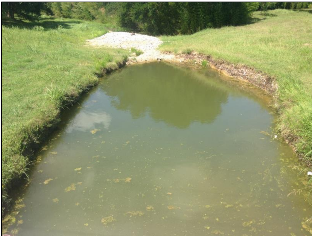
Figure A6. Purgatory Creek below Comal Street; bank erosion and sediment bar, possible due to flow hydraulics of bridge culverts
