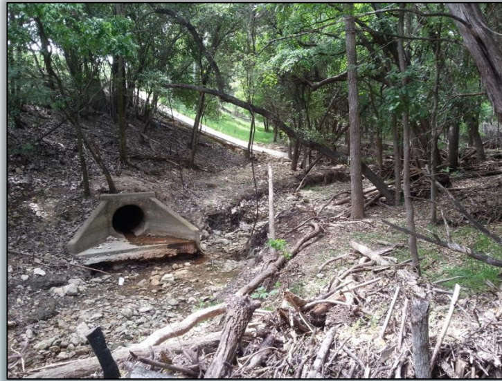
Eroding and erosive outfall from "The Gulch" tributary near RPS project #10 site
