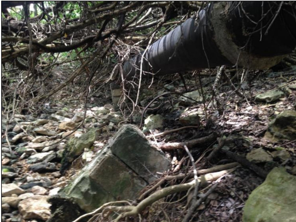
Figure C12. Collapsed wastewater line support in Windmill Tributary
