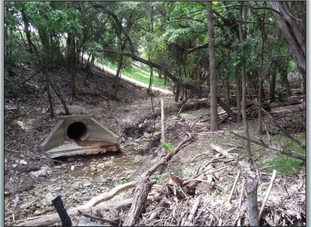
Eroding and erosive outfall from "The Gulch" tributary near RPS project #10 site
