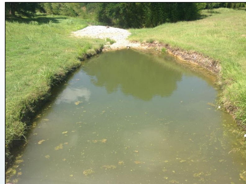
Purgatory Creek below Mitchell Street; bank erosion and sediment bar, possible due to flow hydraulics of bridge culverts
