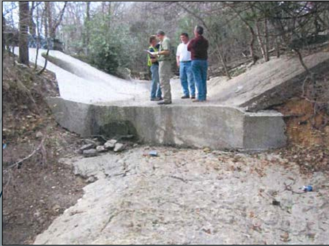
Scour hole below drop structure – Site of RPS project #9 (RPS photo)
