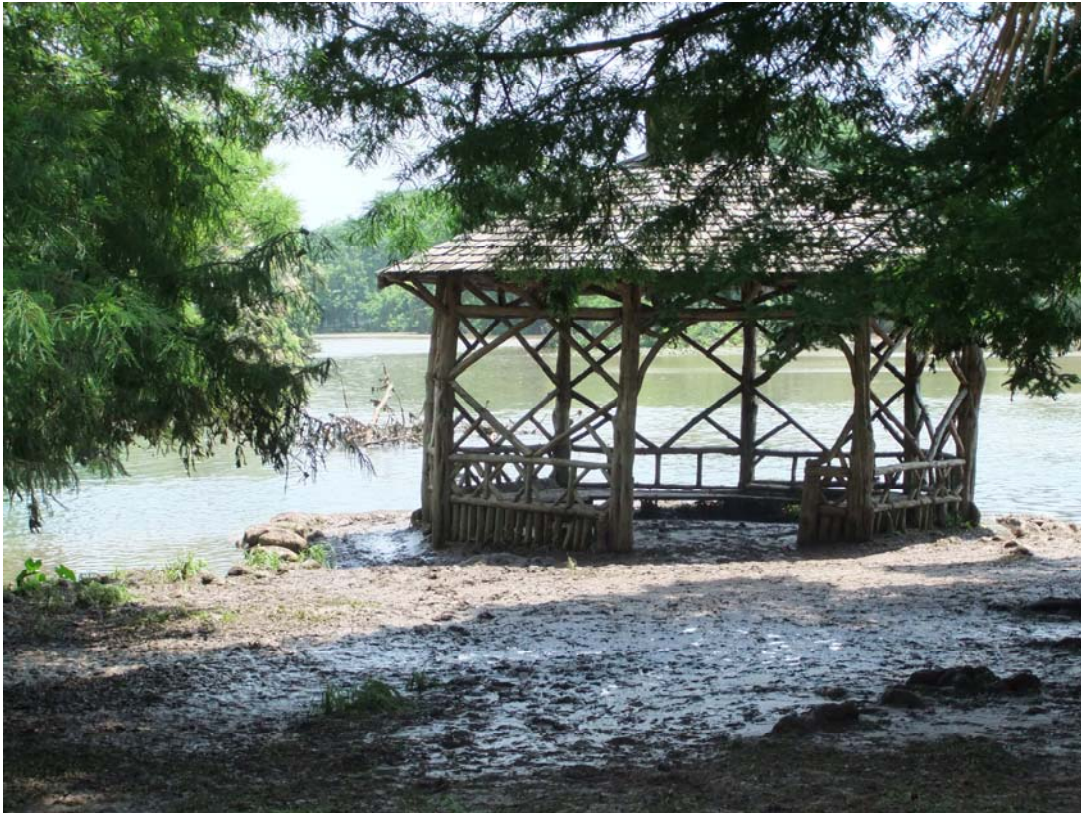
Figure 6. Damage to the gazebo at Landa Lake Park after flood, June 2010.
