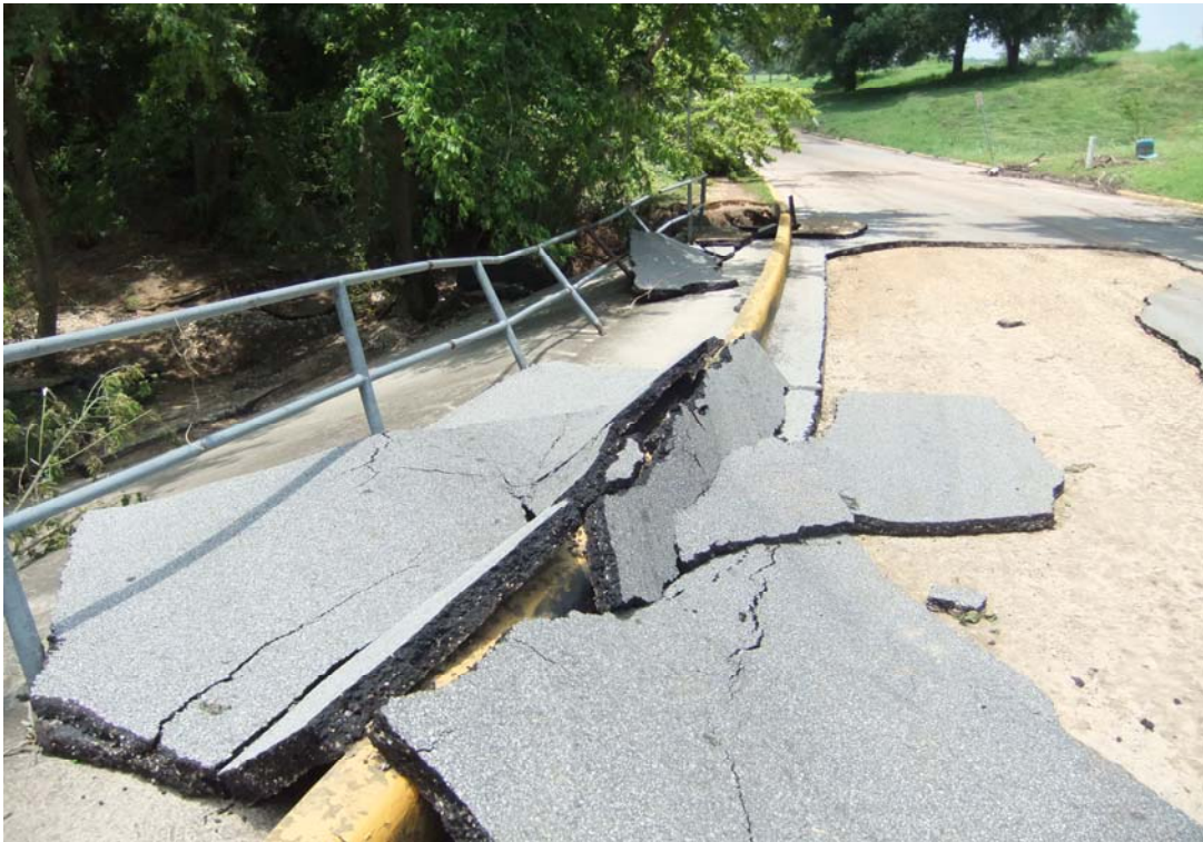
Figure 7. Damage to the Hinman Island Dr. bridge at the Old Channel, June 2010.
