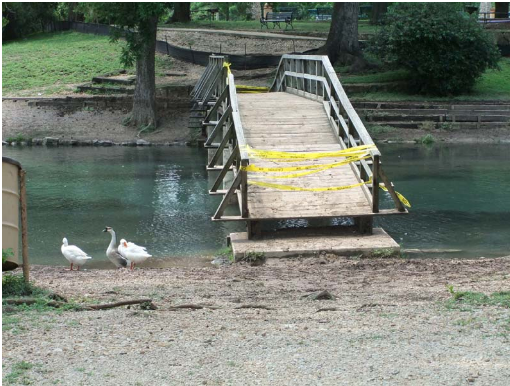
Figure 17. Damage to a pedestrian bridge at Landa Park, June 2010.
